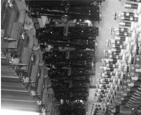
3.13 'Temcooler' active water cooling system fitted to a production draw texturing machine. 27
