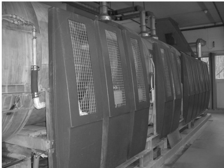
3.54 Industrial laundry equipment with separated chambers.
