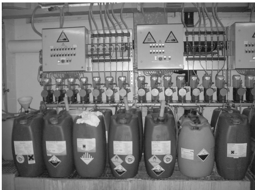
3.47 Automated computer-controlled dosage system for ingredients in wet processing.
