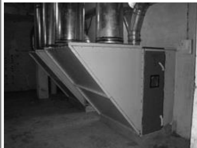
Primary screen filter adopts a rotary filter and continuously filter the air and separated wastes from air
