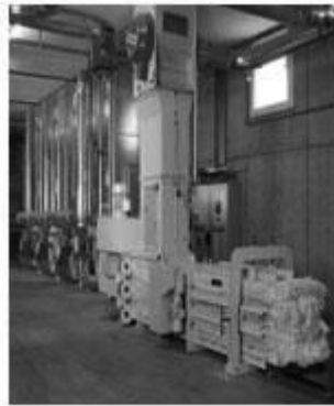
Bale press presses the wastes into compact bales
