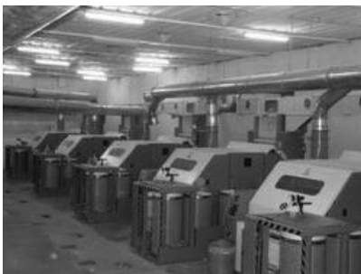
All cards are connected to centralized waste collection unit
